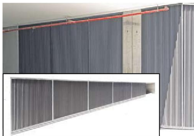
Main & inset picture: ASTL-HE installed at Doha convention centre.
